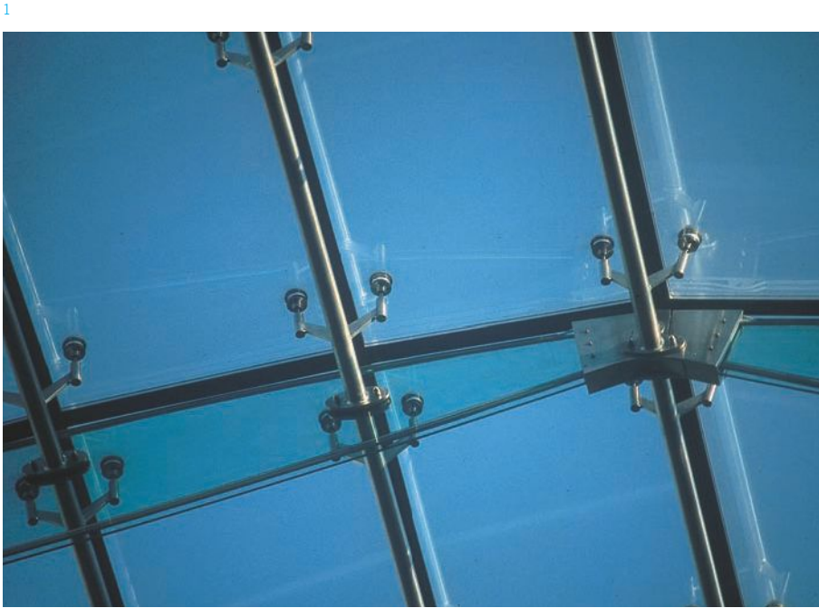
1, 2 The principal load-bearing structure of the roof consists of three-pinned arches, each composed of two laminated glass fins.
